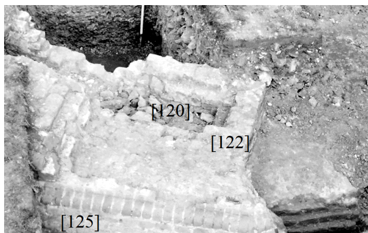
Pl. 34: Tr. D/F, Roofed Section of the Drain (to the Right of [122]), Looking South East
